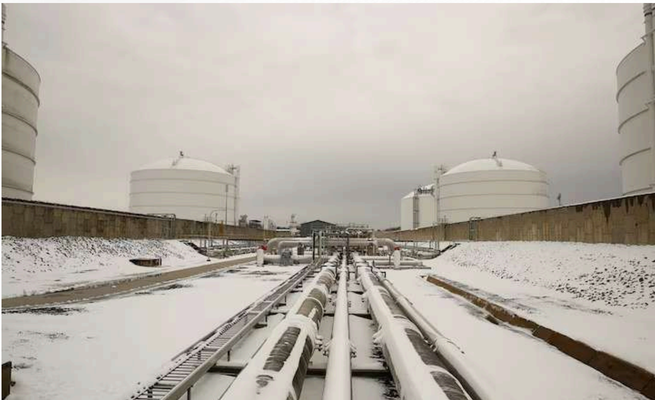
Snow covered transfer lines leading to storage tanks at the Dominion Cove Point Liquefied Natural Gas (LNG) terminal in Lusby, Maryland
