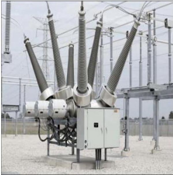
Figure 23: High voltage Circuit Breaker
