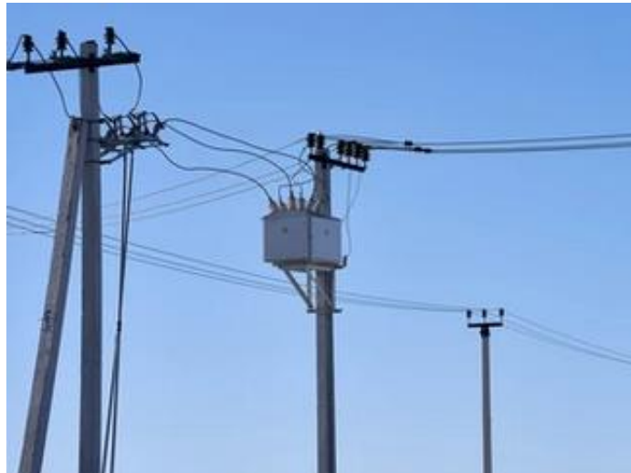
Figure 33: The sub transmission line chuted from main transmission
